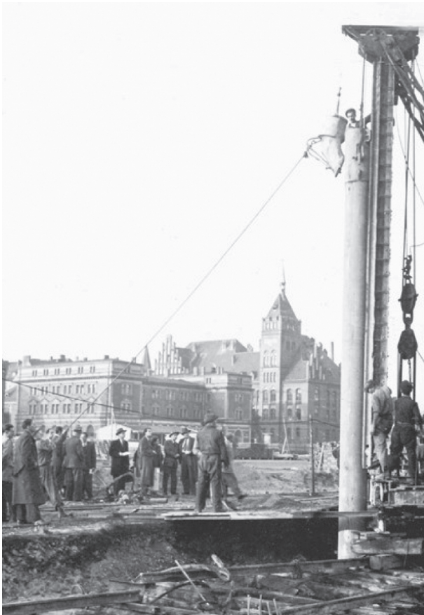
Fig. 3. Beginning of construction of the Faculty of Mining building – embedding of concrete piles
