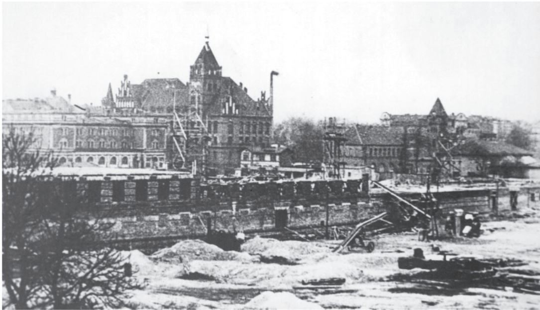
Fig. 2. Beginning of construction of the Faculty of Mining building (view of the Krakowski Square)
