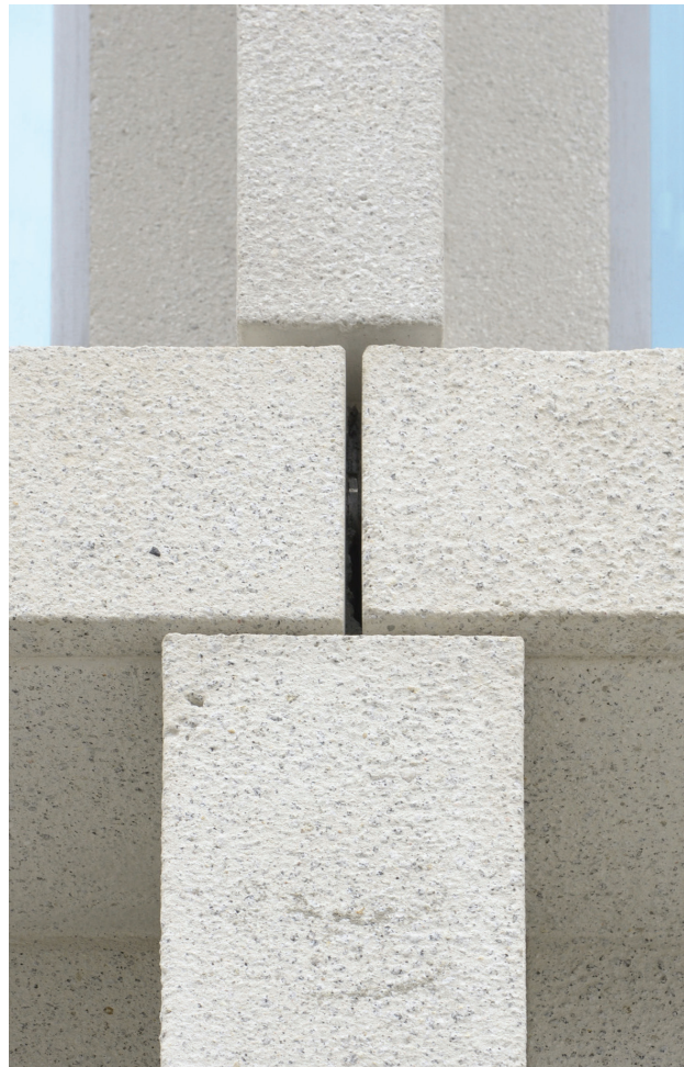
Fig. 9. Wrocław, Nowy Targ Office Building, detail of the concrete façade, designed by Atelier Maćków, 2019 (photo by M. Charciarek)
