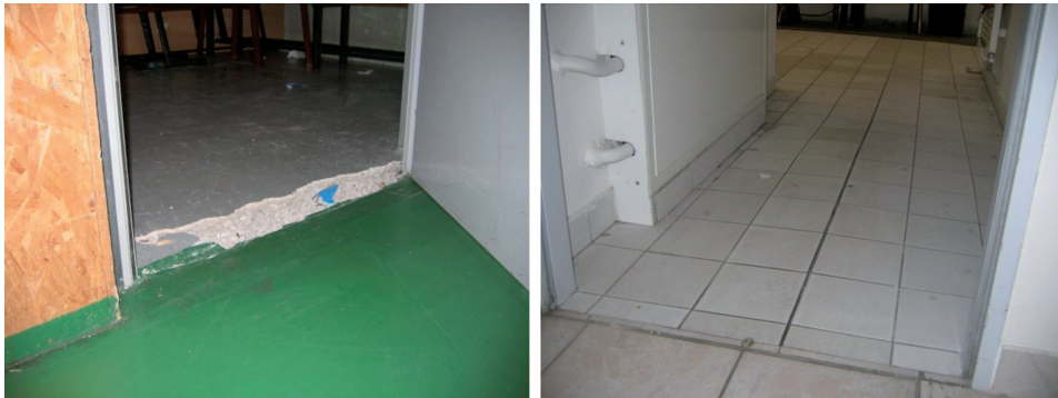
Fig. 4. Threshold failure caused by floor slab lift (left); Visible swelling of the floor with ceramic tiles (right)
