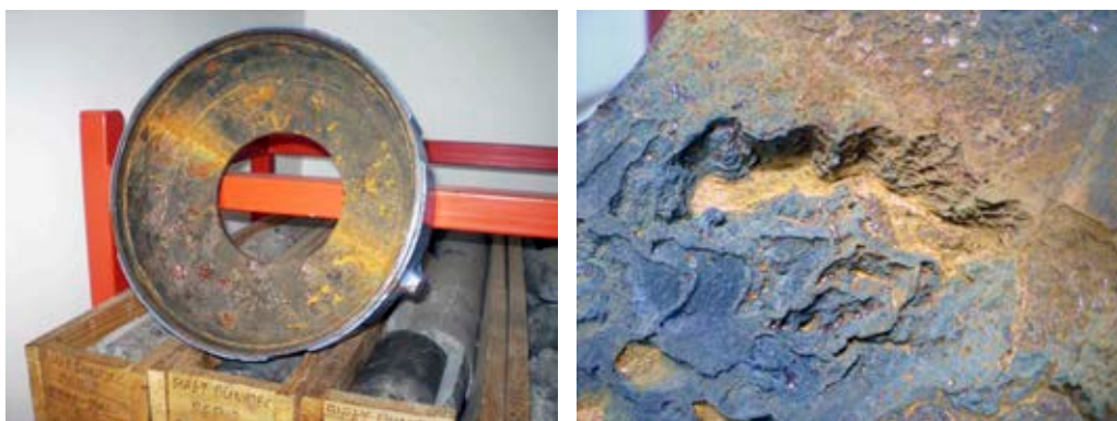
Figure 3. Corrosion damage of a hydromechanical valve component resulting from geothermal water aggressiveness after 5 years of operation in the PGP-1 well
