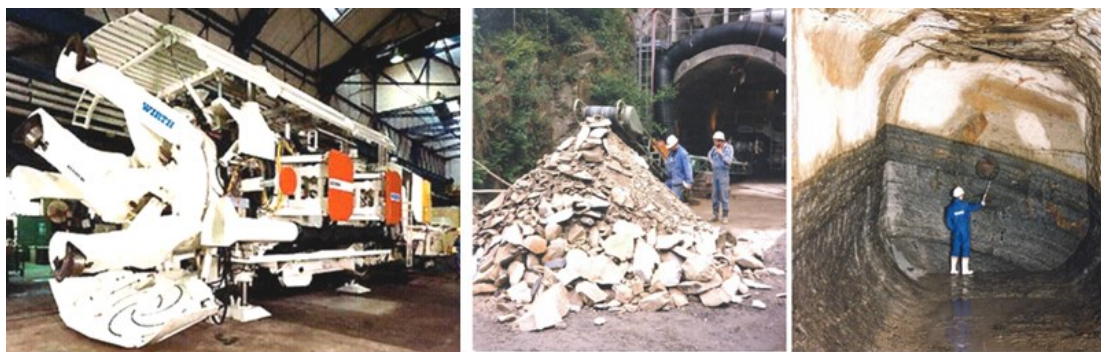
Fig. 3 The view of the Wirth machine used undercutting method and the effects of its work
