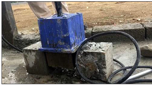
Fig. 1. Water pressure pump
