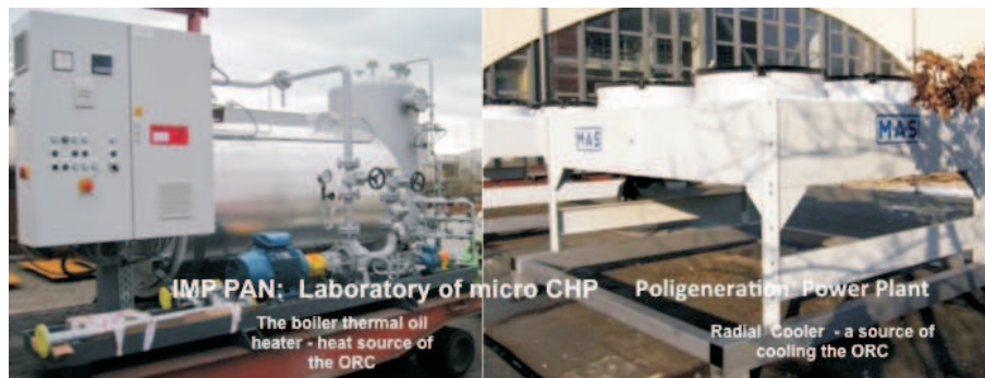
Figure 18: The largest in Poland micro-CHP Laboratory: the poligeneration power plant in the IMP PAN in Gdańsk.
