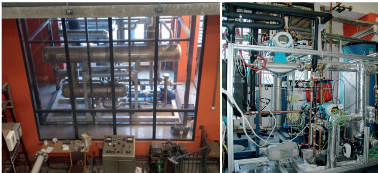
Fig. 2. Micro Power Plant Laboratory situated at the IMP PAN in Gdańsk – ORC installation (on the left) and slide bearings installation (on the right). These installations were used for research on a 100 kW ORC turbine
