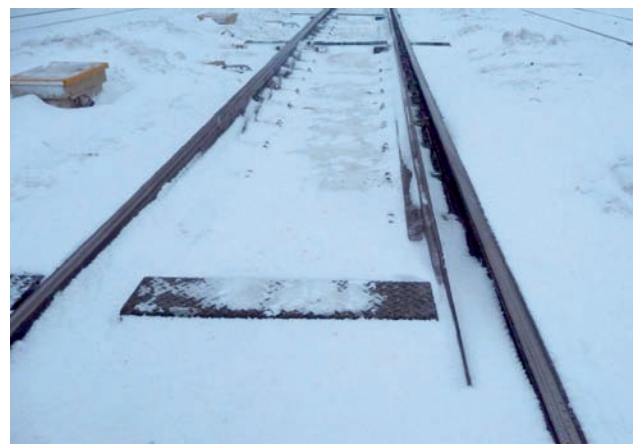
Fig. 3. Inefficient melting out the snow in the switch blade edge zone during intense snowfalls. The visible irregularity of melting out the snow along the stock-rail [PKP PLK January 201]
