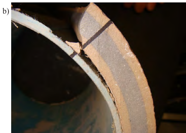
Fig. 10. Samples after the test: a) concrete pipe with liner and b) vitrified clay pipe with liner
