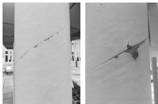
Figure 10. Damages in enamel coating on the columns
