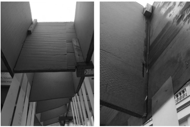
Figure 12. Damages of the cardboard ribs
