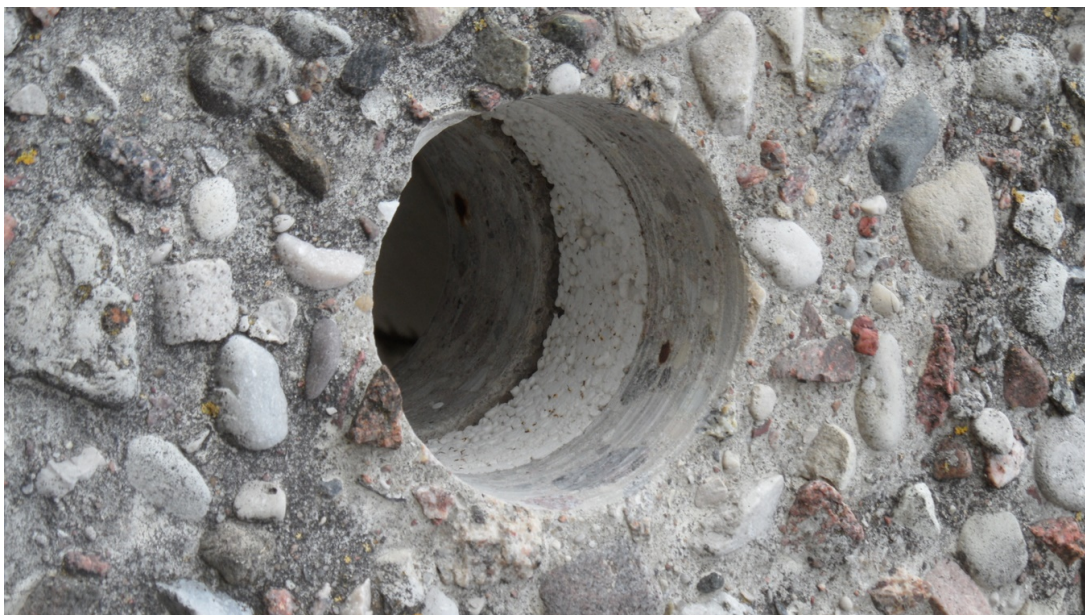
Figure 5. View of the hole made "through" using a drilling rig. [ref. own]
