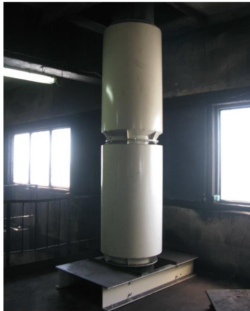
Fig. 5. View of noise silencer of TG type operated in the dust control installation at the coal mechanical preparation plant [9]
