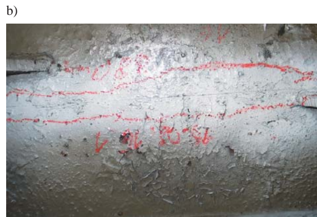
Fig. 3. Cracks of the crane beam revealed by means of the magnetic-powder method: a) type „Z 1 ” joint 120 mm long; b) type „O” plate under the rail, 380 mm long
