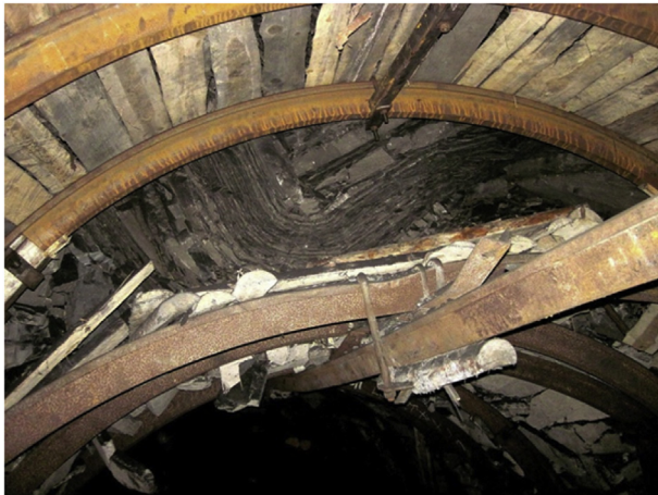
Fig. 9. The wedge of rock extrusion in the conditions of the “Svyato-Andreyevskaya” mine. The 13th Eastern roadway.
