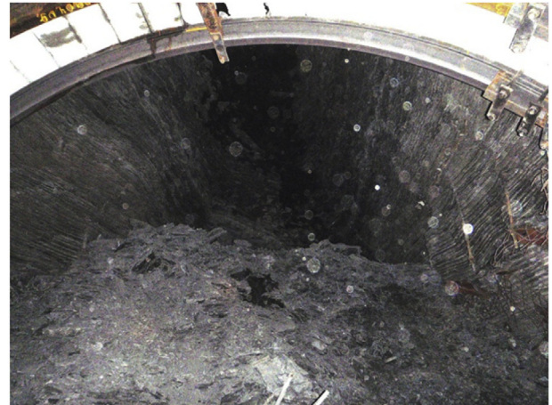
Fig. 11. The roof fall in the 163th roadway in the conditions of the “Stepova” mine.
