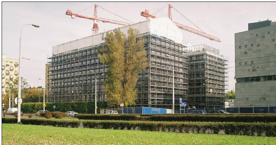
Fot. 1. Biurowiec Green Day we Wrocławiu, Budowa [Wojtyszyn 2013] Phot. 1. Green Day office building in Wrocław, Construction [Wojtyszyn 2013]
