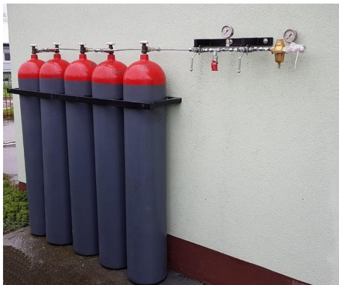
Figure 6. View of the cylinder connection to the biogas supply
