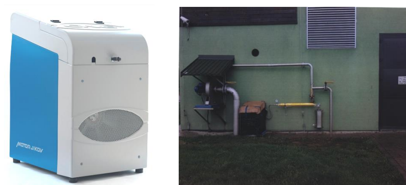
Figure 5. View of the gas installation in the gas compression station. Gas compressor with maximum power consumption of 2.5 kW and a rated capacity of 5 m 3 /h (at 15°C and 200 bar, with an inlet gas pressure of 0.1 bar)
