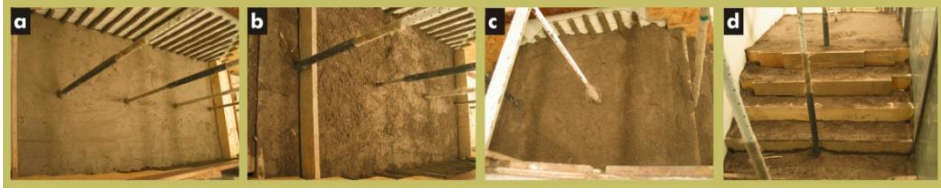
Fig. 2. Formation of a model embankment: preparation of the ground (a), formation and compaction of consecutive layers (b, c), the model before the boarding was taken off (d)
