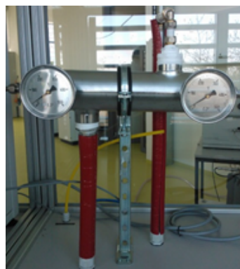
Figure 8. The heat exchanger
