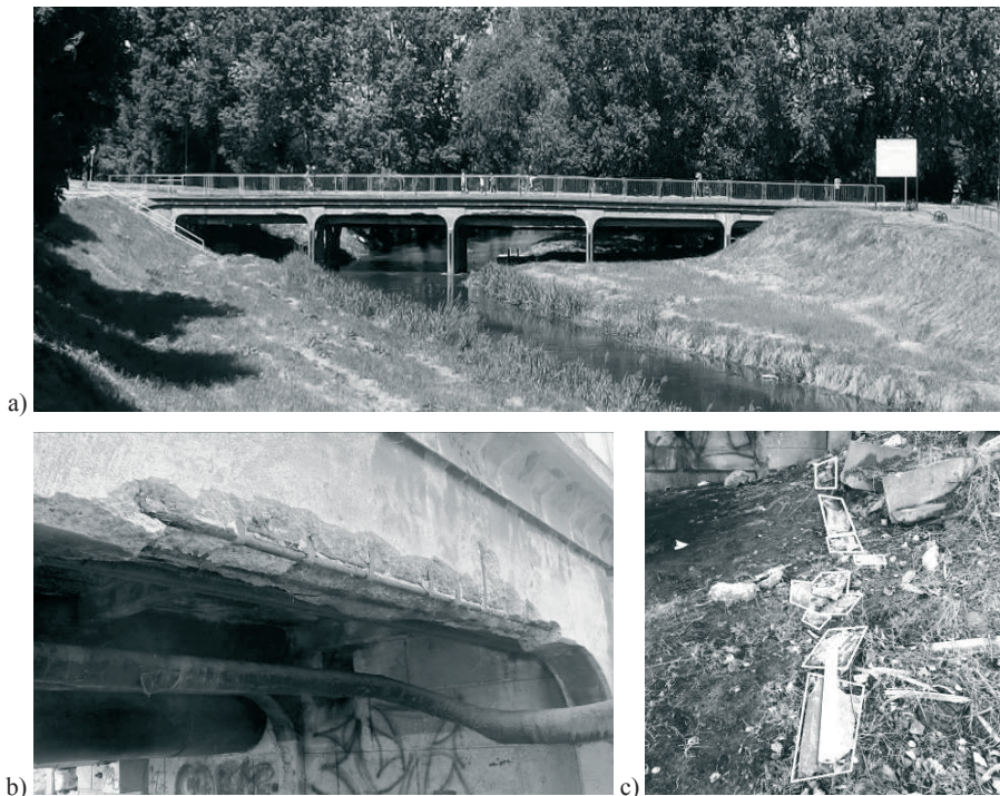
Fig. 2. The 1. Lutosławski Bridge in Kalinowszczyzna, Lublin a) side view b) outer beam corrosion c) fresh peeling of concrete cover of reinforcement (photos b-c were taken on 03.03.2016)
