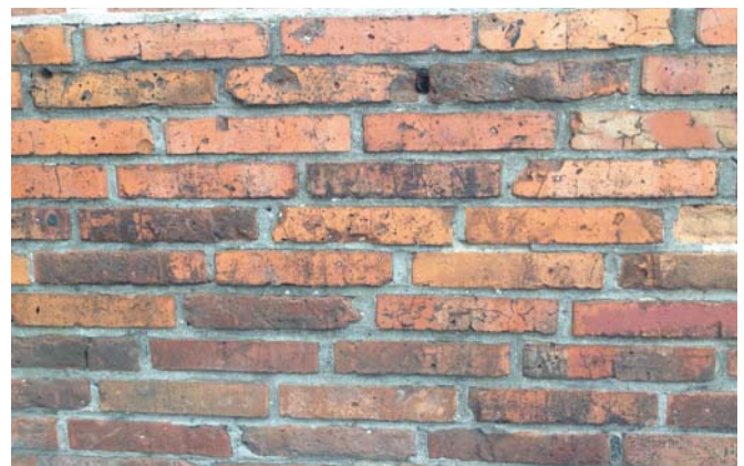
Fig. 11. View of both serviceable and damaged brick wall structure
