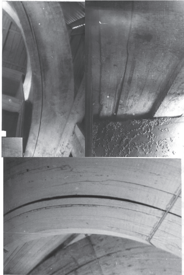
Fig. 1. Fragments with cracks passing in the GLBF from the ledge in the crossbar to the support
