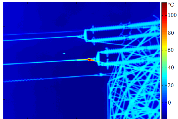
Fig. 1. The exemplary thermogram of a power line
