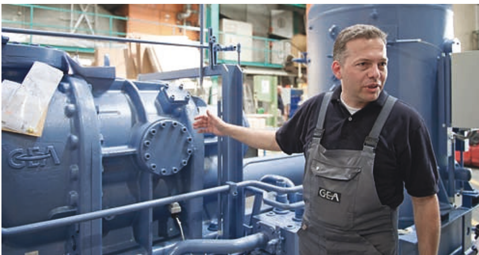
Fig. 3. "Thanks to the high-precision manufacturing processes, the screw compressors from GEA Refrigeration Germany are very energy efficient," explains measuring technician Carsten Göbel
