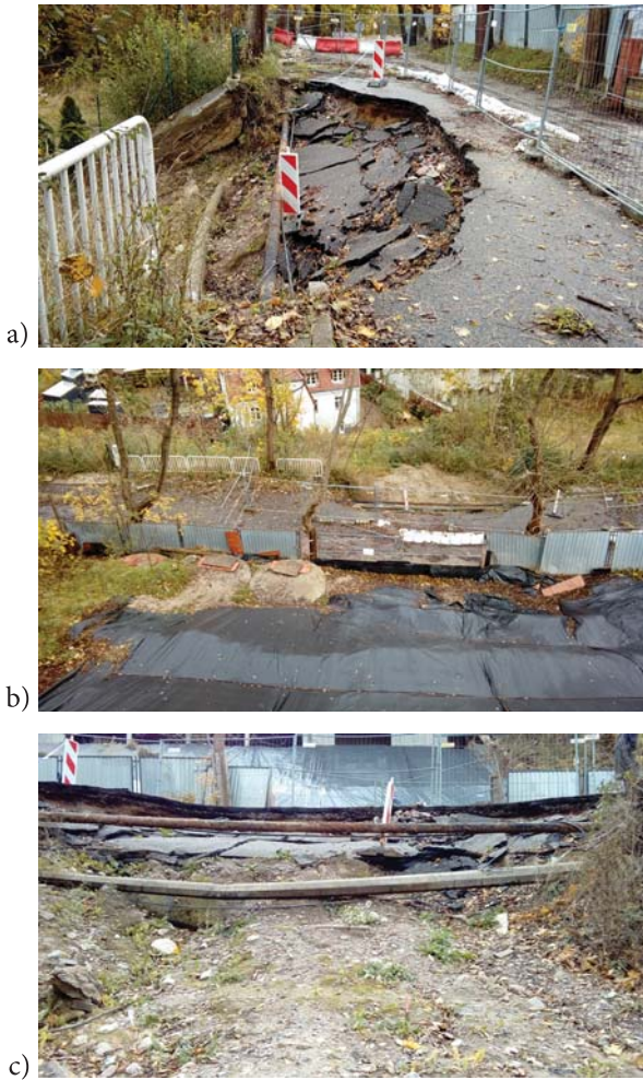
Fig. 5. State of the landslide 8 months after the damage
