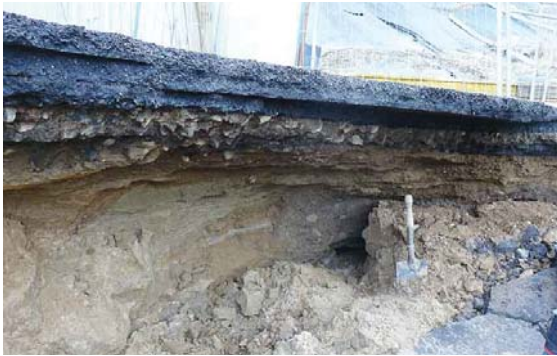
Fig. 4. A cavern and hydraulic piping flow canal revealed after the damage [10]
