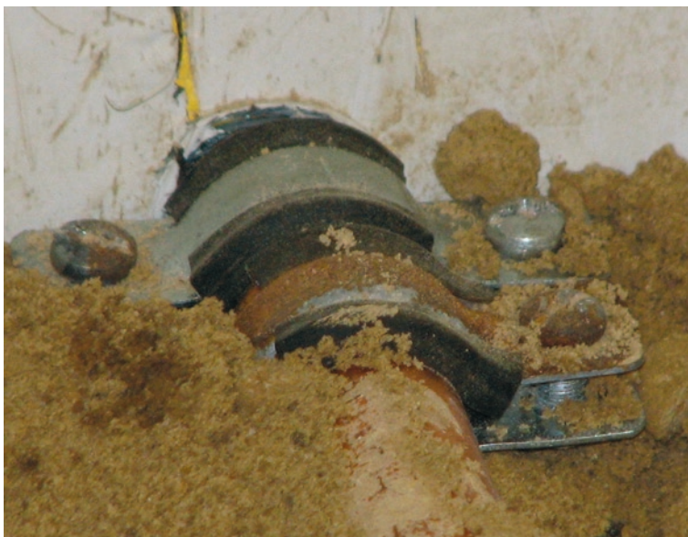
Fig. 2. Holder enabling the same width of leak after each loosening of pipe connection
