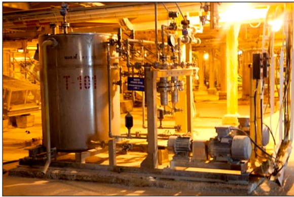
Fig. 4. Inside the sulfur granulation complex at the Astrakhan gas processing plant
