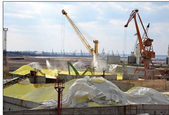
Fig. 9. Construction of a complex for reloading industrial sulfur in the sea port
