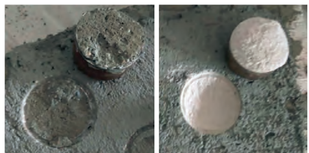
Fig. 11. Damage during adhesion tests on notched samples of concrete (left) and aerated concrete (right)
