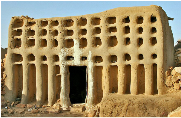
Fig. 6. Adobe buildings – a ‘gina’ (highhouse) of the Dogon people of Mali (Sangha, Mali), built with Sahelian adobe
