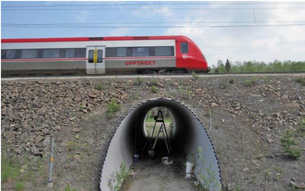
Fig. 1. Sample soil shell structure made of corrugated sheets used as a railway culvert
