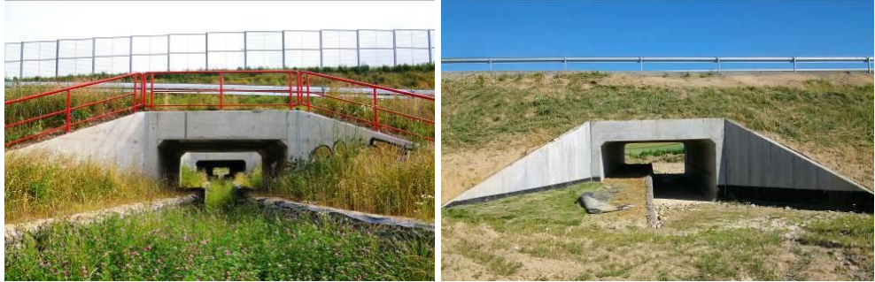
Fig. 1. The solution for animals crossing in the form of shelves with gabions in the facility PZM 33
