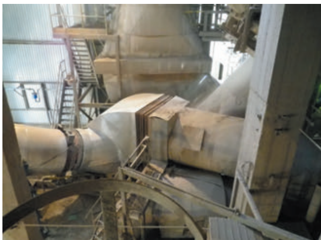
Fig. 2. Real condition on site – gasses distribution
