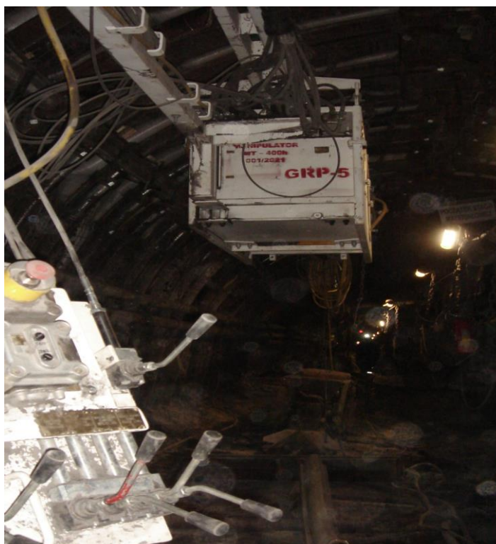
Fig. 11 The modular installation and transport assembly at the site of arch support frame installation
