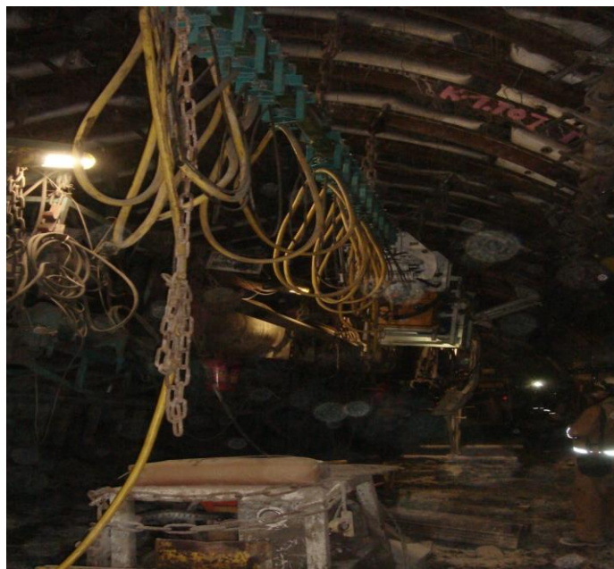
Fig. 10 The modular installation and transport assembly in the support elements storage area
