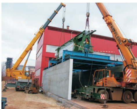
Photo. 4. Installation of the technology of the dry refrigerant system Source: photo taken by the author.
