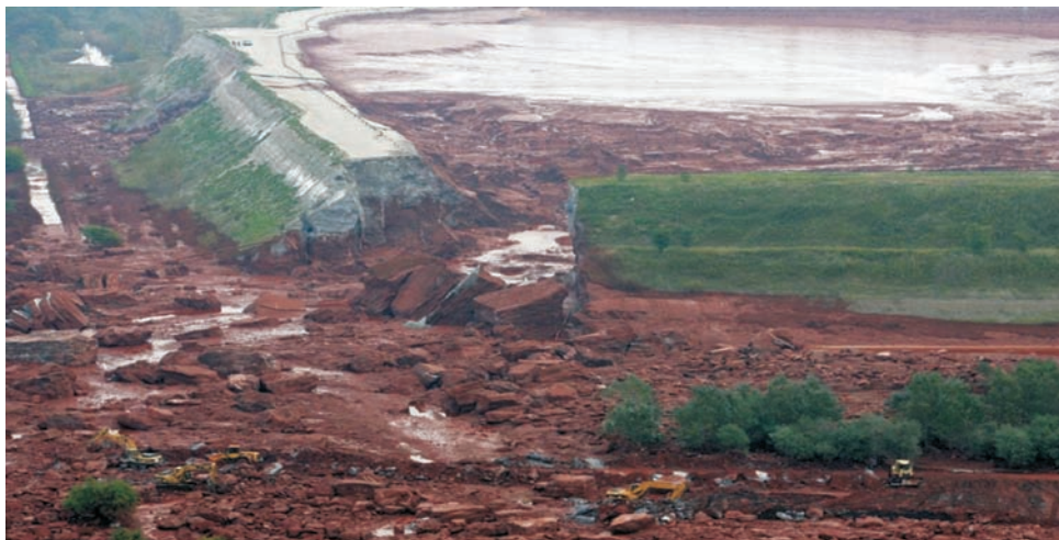
Photo. 1. The broken dam (outside view)
