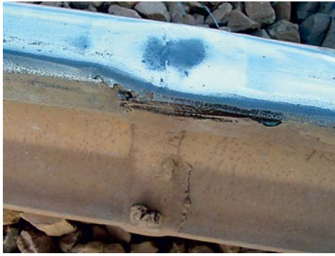
Rys. 10. Wada na złączu spawanym termitowo oznaczenie 422 Fig. 10. Defect on the termite welded joint designation 422
