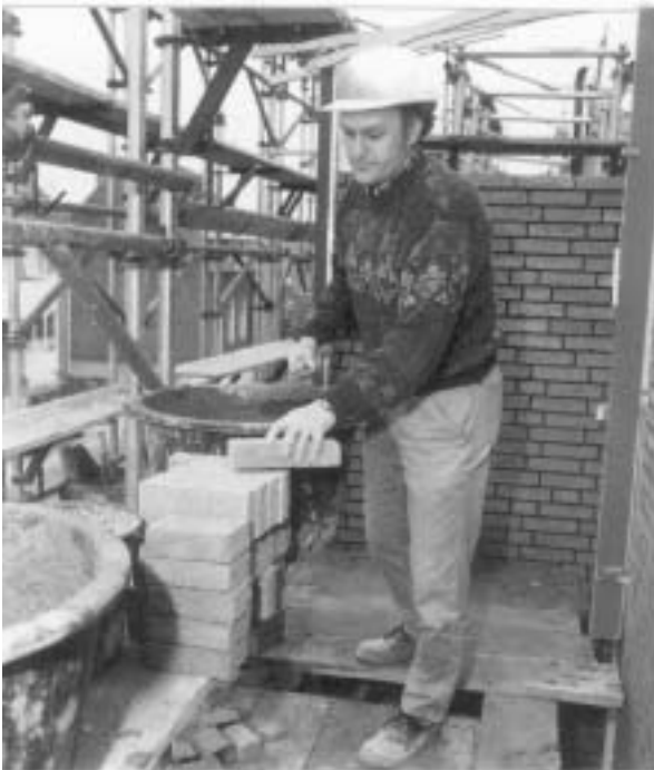
Figure 2. Bricklaying with a split floor scaffolding with bricks and mortar 50 cm raised.
