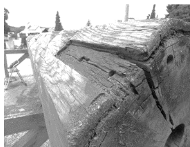
Fig. 2. Damage to monument due to the fastening system
