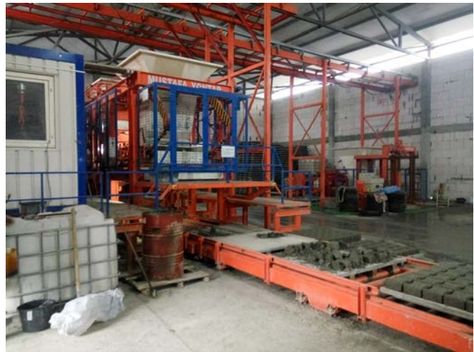
Fig. 1. View of ICB production equipment
