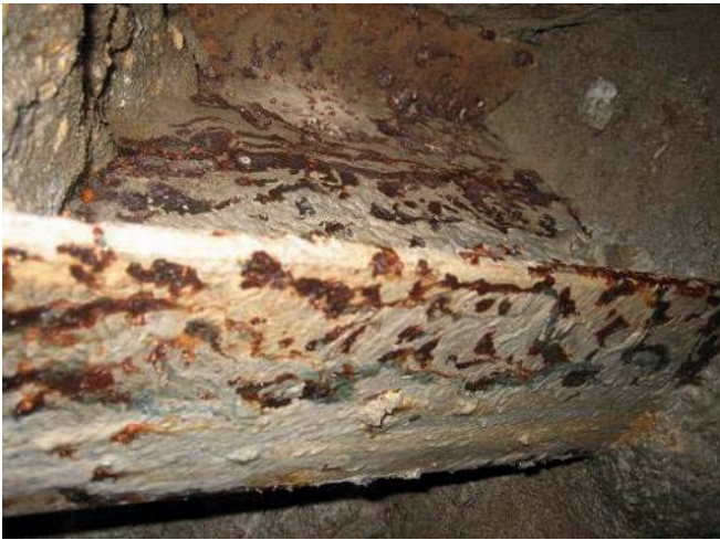
Fig. 8. Steel corrosion in primary support of subsea tunnel
