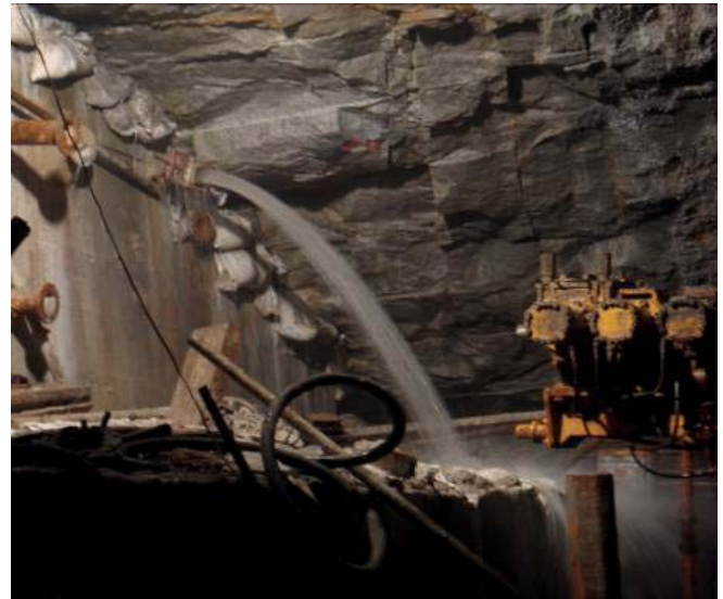
(a) Large amount of water in tunnel before grouting
