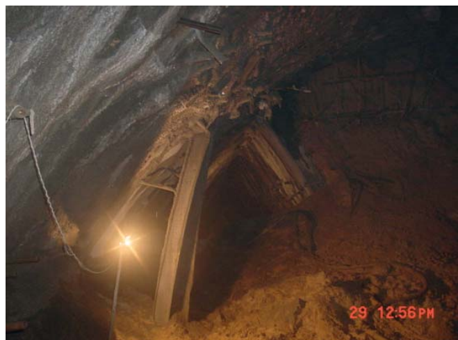
Fig. 5. Intrusion of surrounding rock and primary support in clearance limit of subsea tunnel
