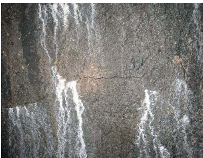
(b) Cracking and water seepage of primary support
