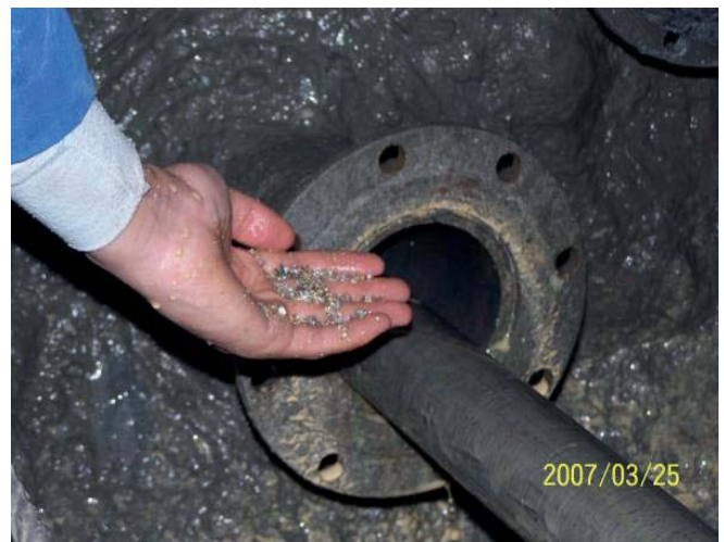
(b) Tunnel water disappeared after grouting
