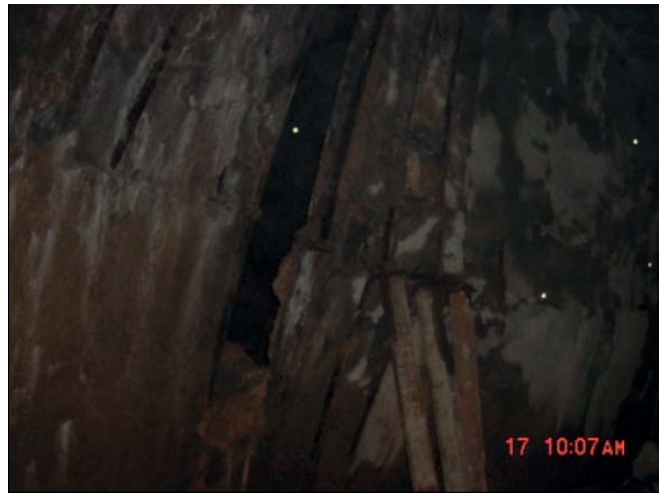
Fig. 4. Concrete peeling and steel arch distortion of primary support in subsea tunnels
