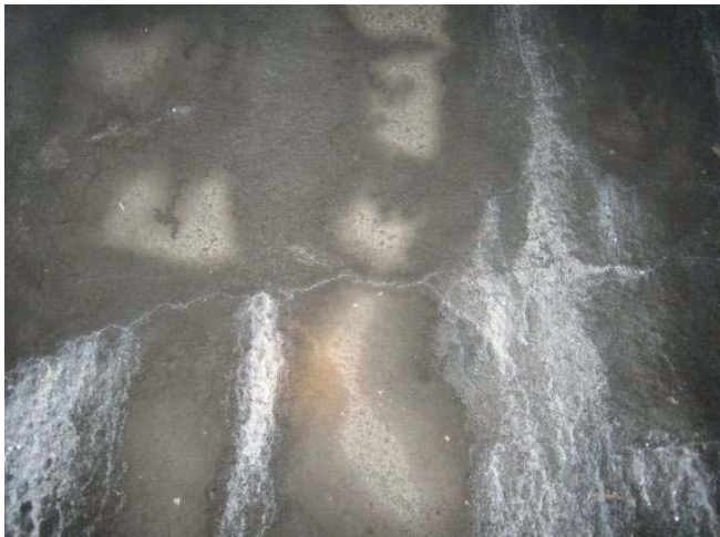
(a) Cracking and water seepage of primary support
