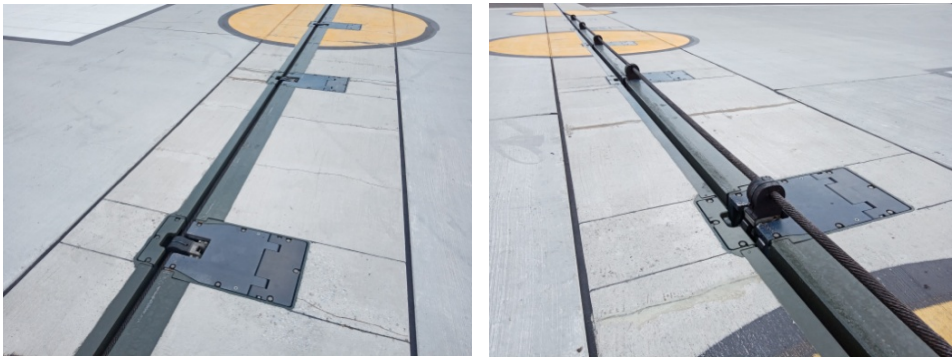
Fig. 5. BAK-12 system with the retractable arresting cable - airfield in Łask in Poland
