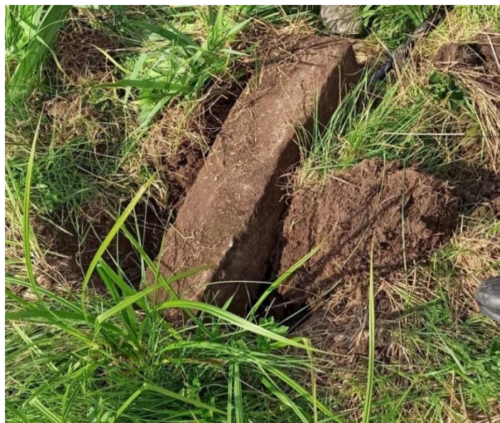
Figure 4. An example of a damaged control network point found during a field interview. Source: the authors' archive.
