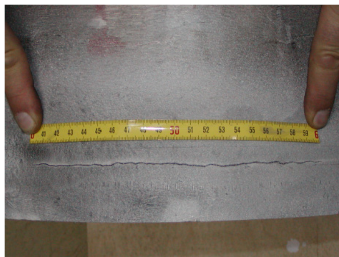
Fig. 1. The main crack - a view from the outer side in the place of the welded joint
