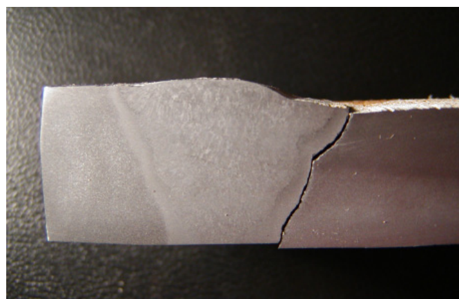
Fig. 2. The main crack from the pipeline's side extending through the HAZ – a cross section
