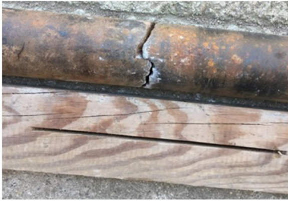
Fig. 29. The shaft broken by bending under the effect of static deformation and fatigue
