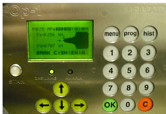
Fig. 15. Operator panel with screen
