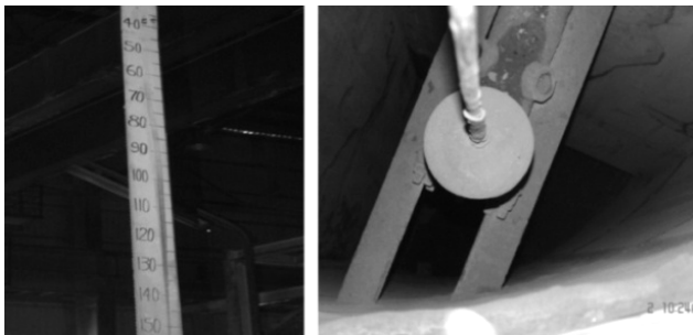
Fig. 6. Installed float near the column
