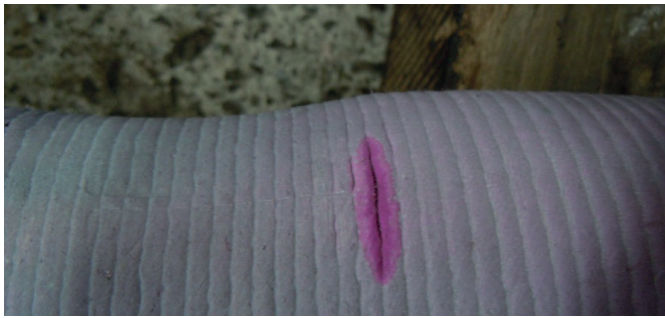
Fig. 16. An indication of the crack after PT on the singular pipe spirally surfaced by welding
