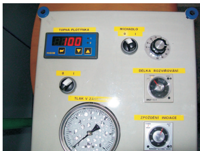
Fig. 1. Operator control unit with HT60B
