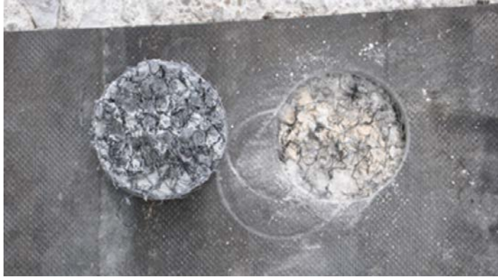
Fig. 10. Failure between the plastic hook-and-loop-like anchor layer and the concrete surface of the sleeper (failure type A/B)
