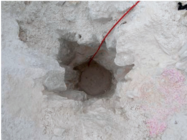
Fig. 3. Cracked hole collar and hardened plaster
