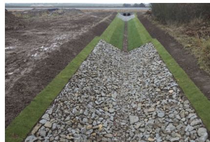
Fig. 8. Example of a proper solution strengthening the watercourse using stone material and turf
