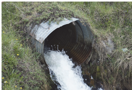
Fig. 3. An example of the local surface corrosion of corrugated steel shell structure in the bottom area (example from South Argentina)
