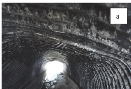
Figure 4a. Example of damaged steel shell structure built as culvert within highway during its construction
