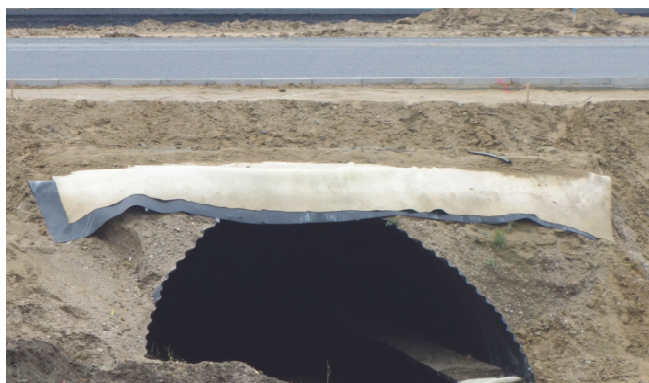
Fig. 13. Example of additional reinforcement of flexible corrugated steel shell structures with geotextile built in the upper zone of backfill.
