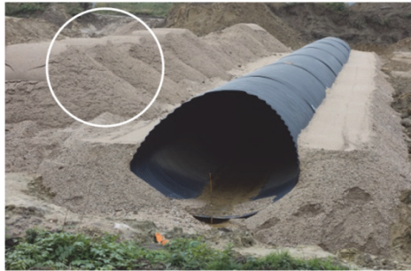
Fig. 11. Example of the initial stage of backfilling of a flexible corrugated steel culvert structure. An inadequate size of backfill in the side zone of the structure can be seen
