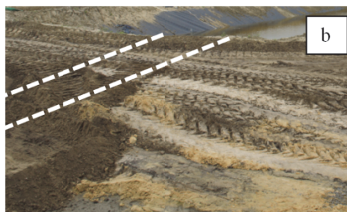
Fig. 4b. Visible inappropriate conditions of soil backfill over the structure (cohesive soil, too low thickness of backfill with intensive construction-site traffic)
