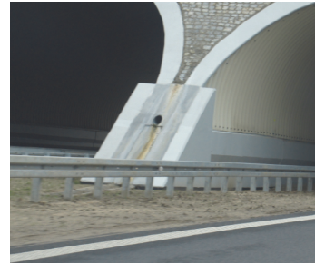
Fig. 6. Example of leakage on the front wall around the middle support area of an eco-bridge
