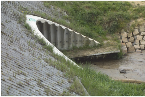
Fig. 9. Example of shelves for animals in a complex functional culvert. An erosion of soil surface on the shelf and the corrosion of the shelf structure can be seen
