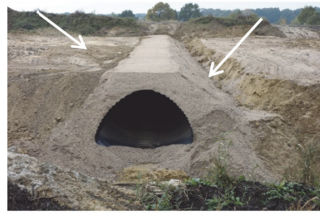
Fig. 12. Example of backfilling of a flexible corrugated steel culvert. An unbalanced embankment resulting from horizontal deformation of the steel shell structure can be seen
