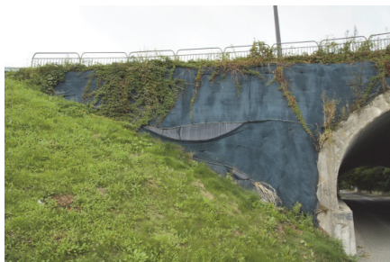
Fig. 7. Example of improper protection of slopes using geotextile in corrugated soil-shell structure in service
