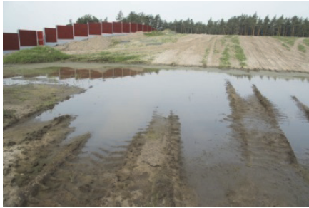
Fig. 5. Example of hollows of water on the soil surface of the eco-bridge situated above the main railway line and expressway
